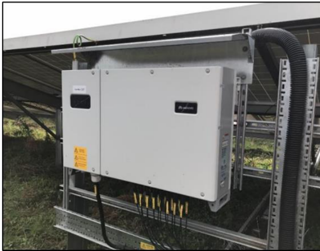
Plate 2.1: Typical String Inverter
