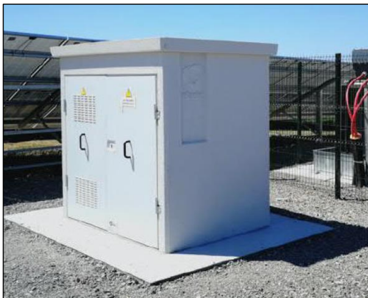
Plate 2.4: Typical outdoor switchgear
