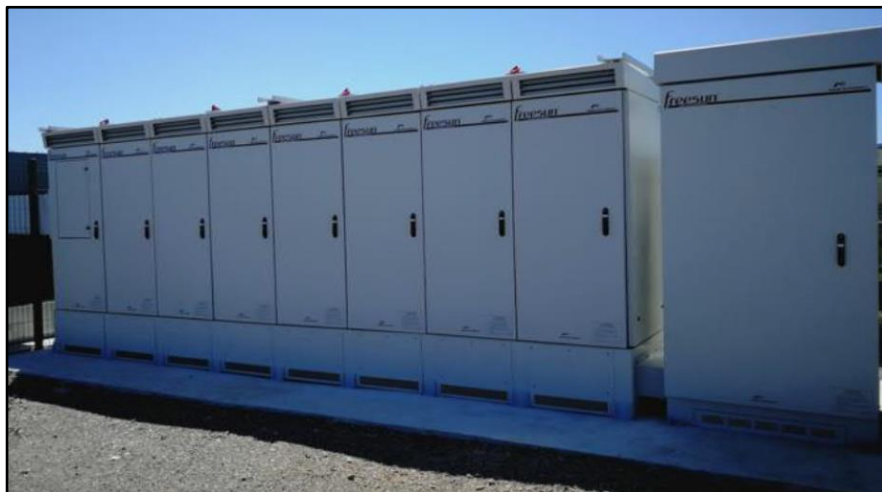
Plate 2.2: Typical Centralised Inverter
