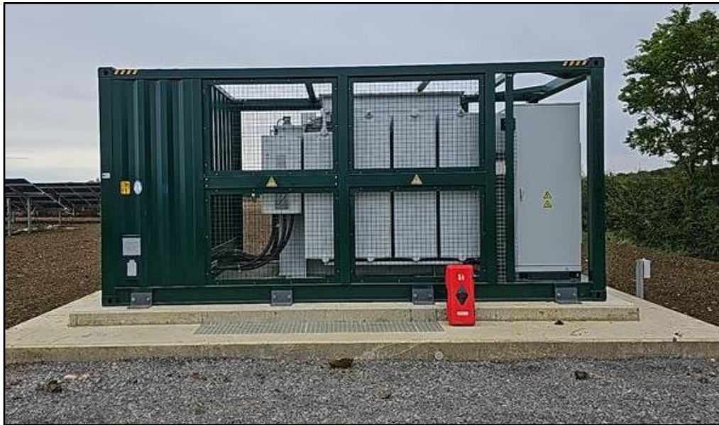
Plate 2.3: Typical outdoor transformer
